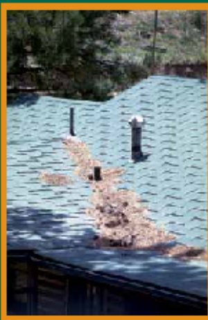
Figure 15: Clearing pine needles and other debris from the roof and gutters is an easy task that should be done at least once a year. Photo: CSFS
