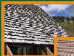
Figure 8: (above) Wood shingle roofs are highly flammable and not recommended. Photo: CSFS
